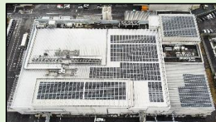
Ryugasaki Frozen Food Plant Photovoltaic power generation facility
